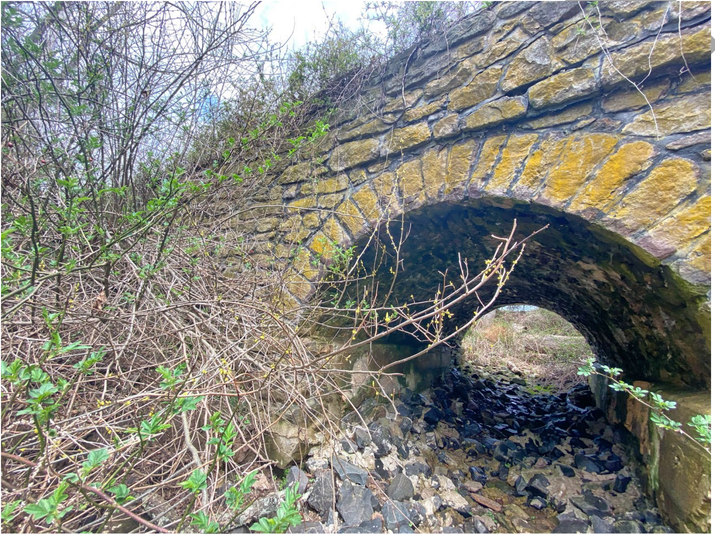
Photo 7: Southwest (downstream) side of the bridge, view facing north showing the southwest wingwall
