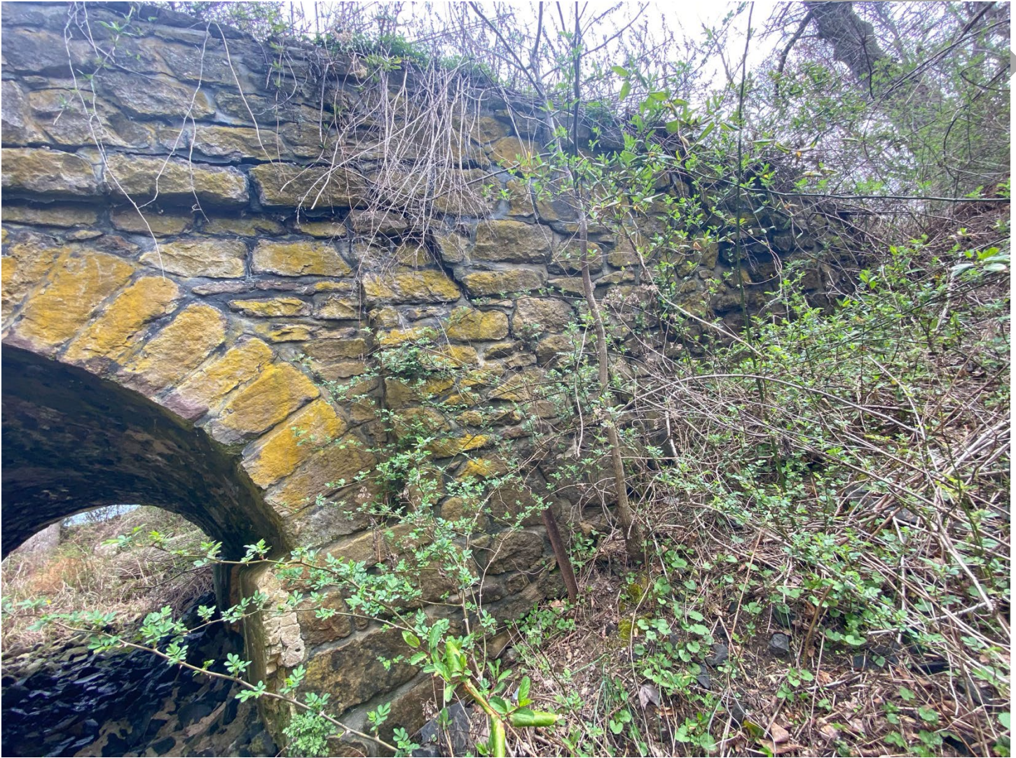
Photo 8: Southwest (downstream) side of the bridge, View facing northwest showing the southeast wingwall
