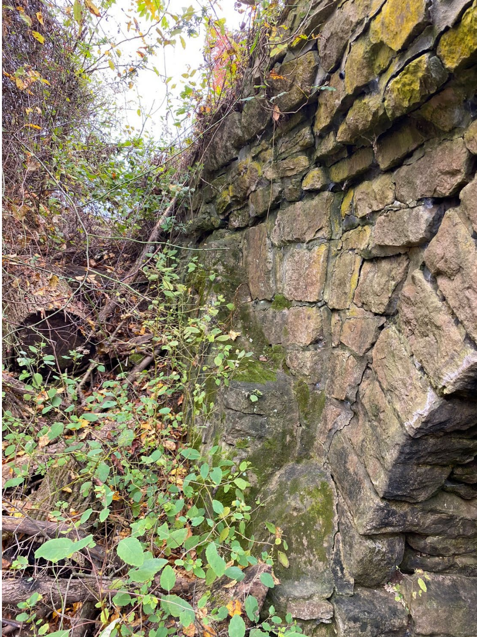
Photo 4: Northeast (upstream) side of the bridge, view facing south showing buttress at the base of the northeast wingwall, the arch ring, spandrel, and the displaced parapet.
