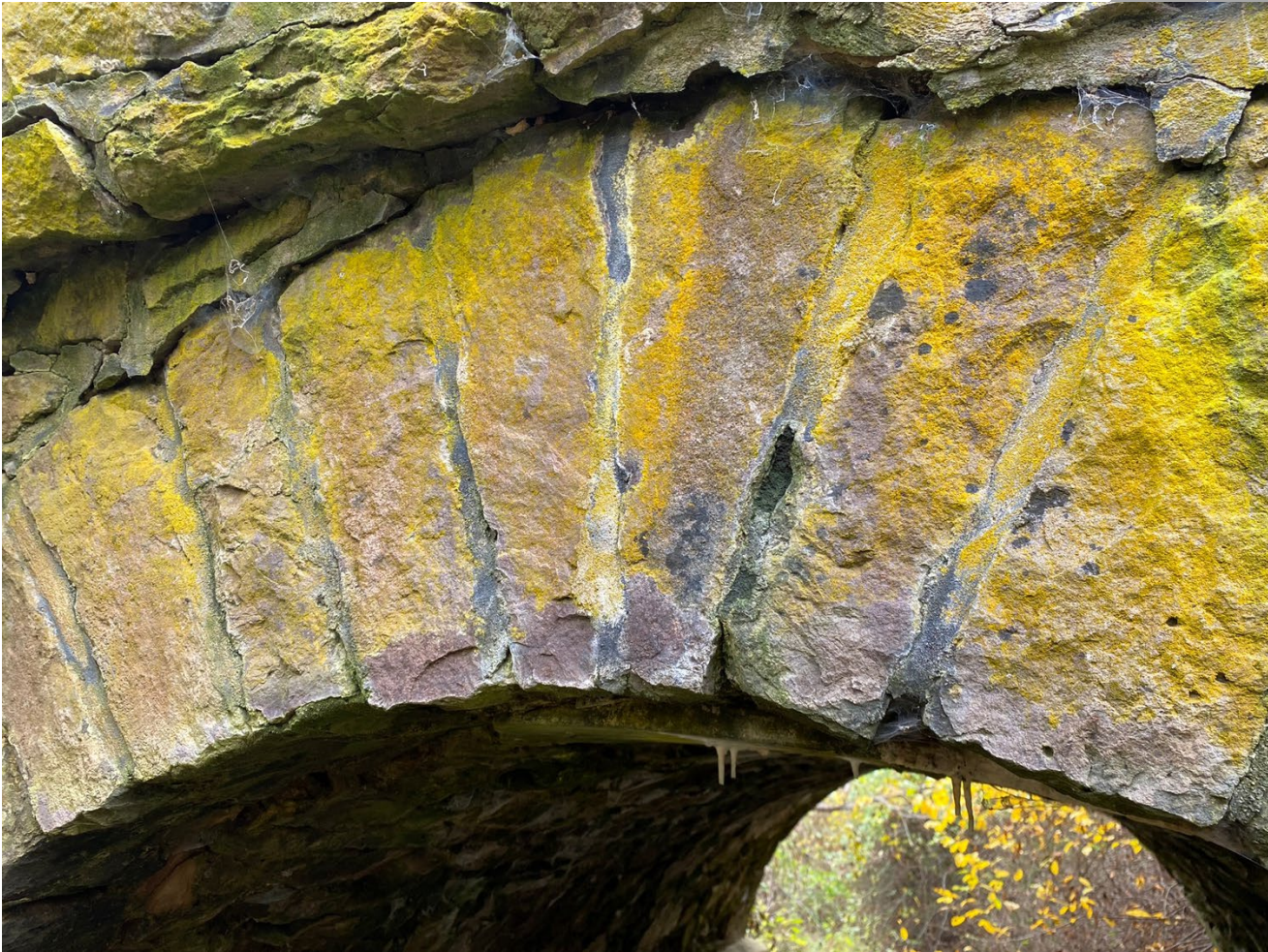
Photo 5: Northeast (upstream) side of the bridge. View facing southwest showing the split keystone and the cantilevered parapet wall.
