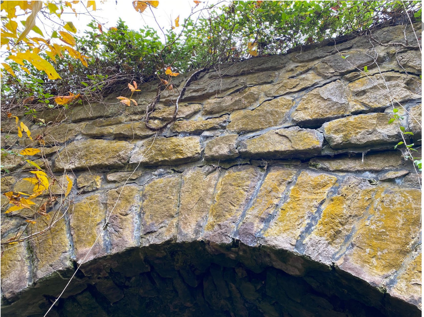
Photo 9: Southwest (downstream) side of the bridge, view looking up at the apex of the arch ring and the cantilevered parapet.
